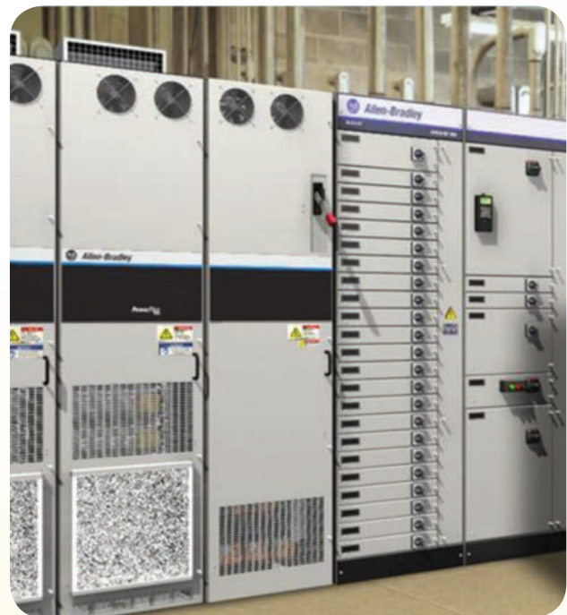
Continuous, side by side installation of PowerFlex 755 floor mount drives and MCCs helps to reduce the number of mechanical components and lessen floor space requirements.
